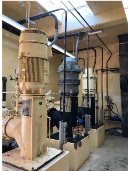
Effluent pumps 1, 2, and 3
