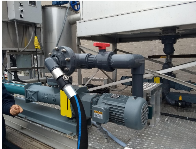
WAS Progressive Cavity Pump
