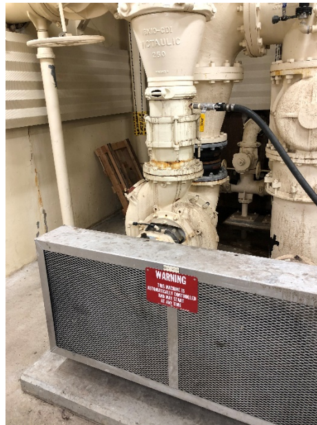
Existing sludge mixing pump 2
