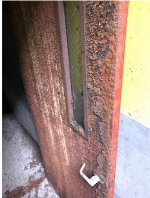
Wet well door
