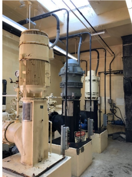
Effluent pumps 1, 2, and 3
