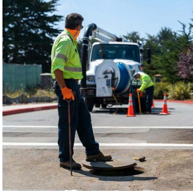
Sewer flushing truck in service
