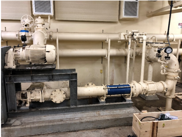
Progressive cavity sludge feed pump
