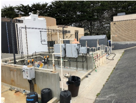
New chemical feed pumps and controls
