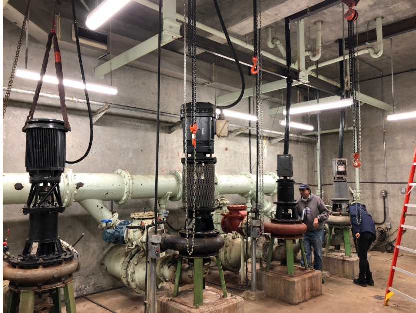
Pumps 1, 2, 3, and 4 (from left to right)
