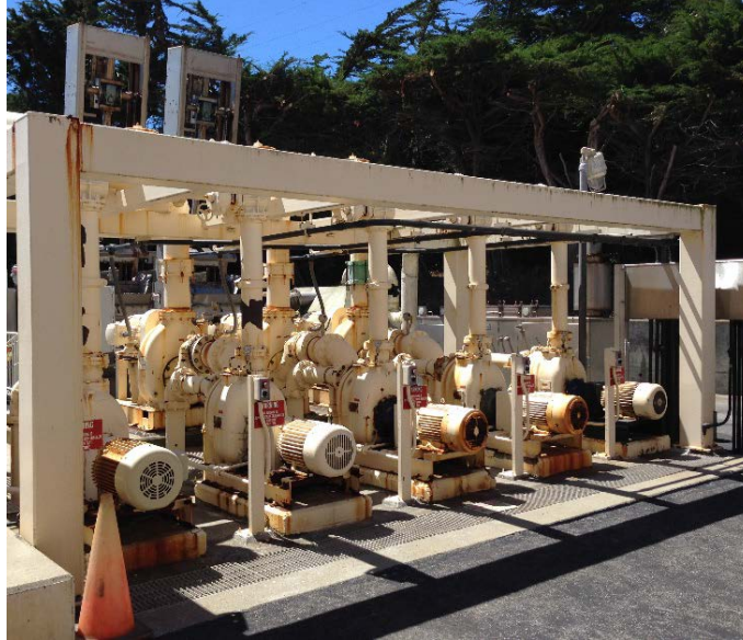
Influent Pump Station
