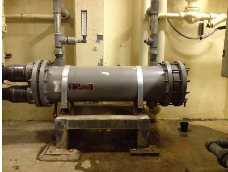
Existing heat exchanger
