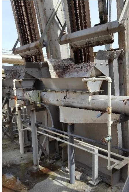
Automatic bar screens 1 and 2
