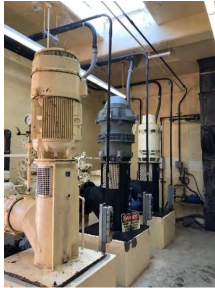
Effluent pumps 1, 2, and 3
