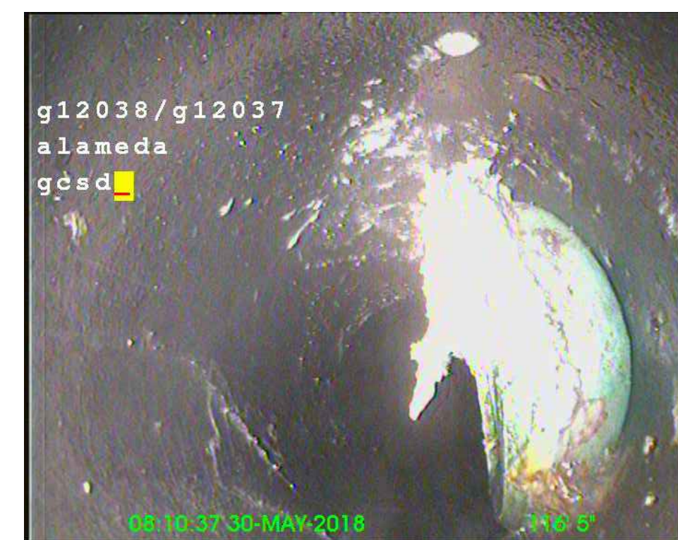
(E) PROTRUDING LATERAL
