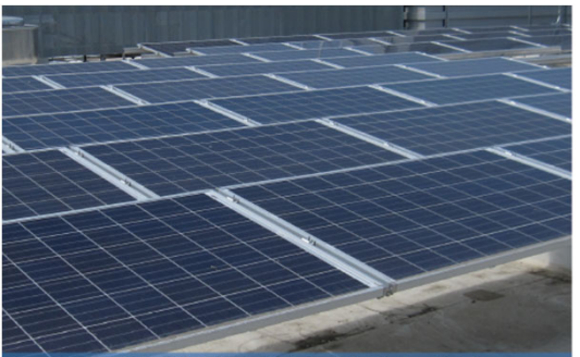
ROOFTOP SOLAR PANELS
