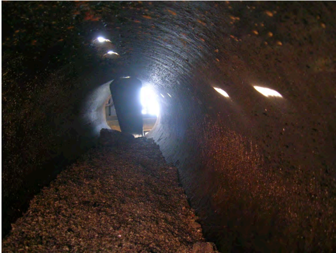
Figure 5 Pipe Damage and Grit
