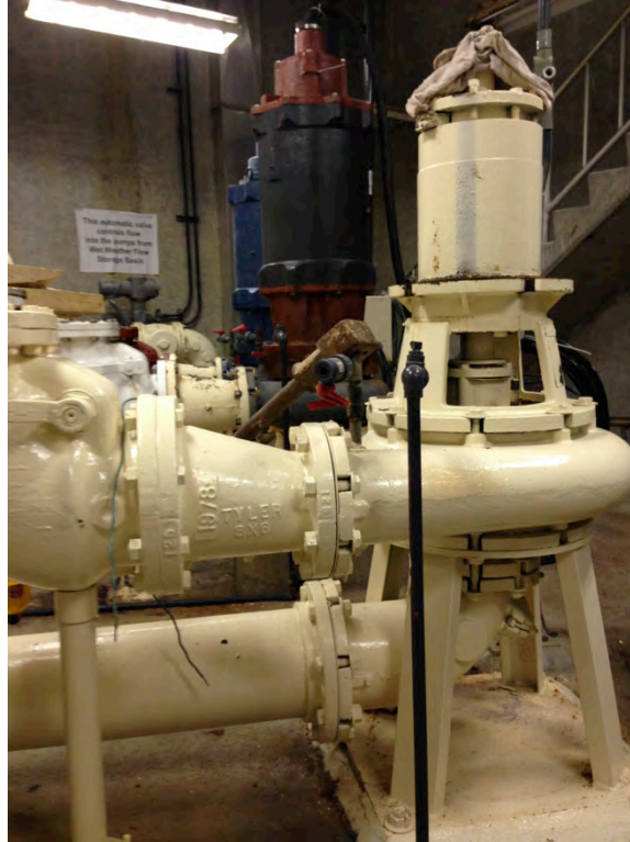
Figure 2 Montara PS Small Pump – Non-Operational
