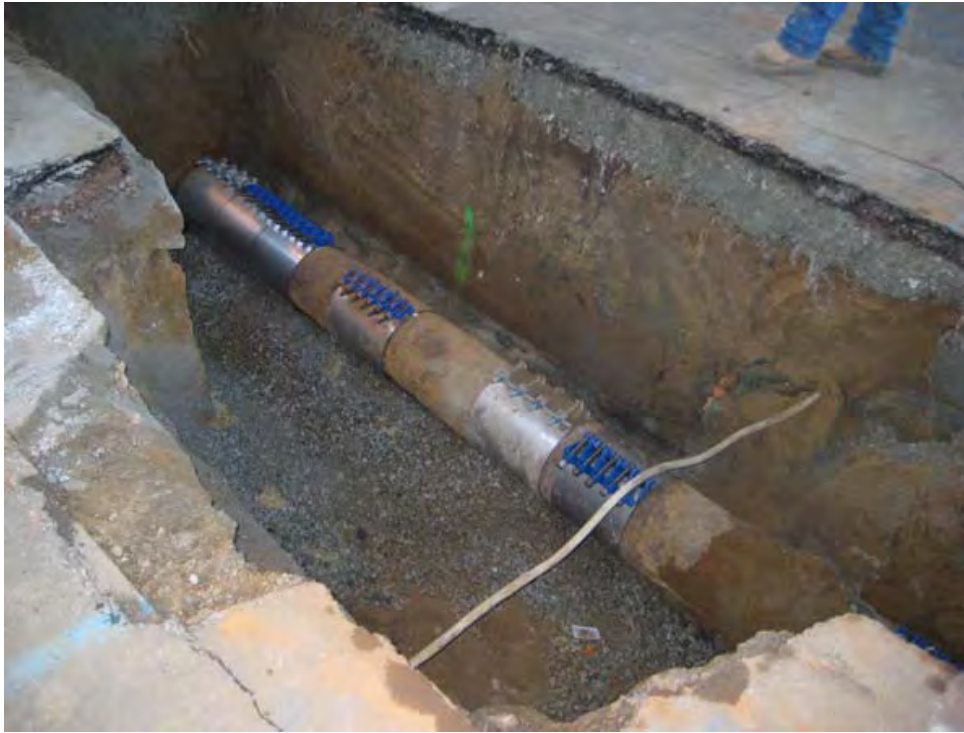
Figure 7 Six Repair Clamps Within About 10 Linear Feet of FM
