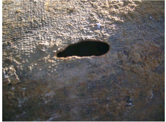
Figure 6 Pipe Wall Damage
