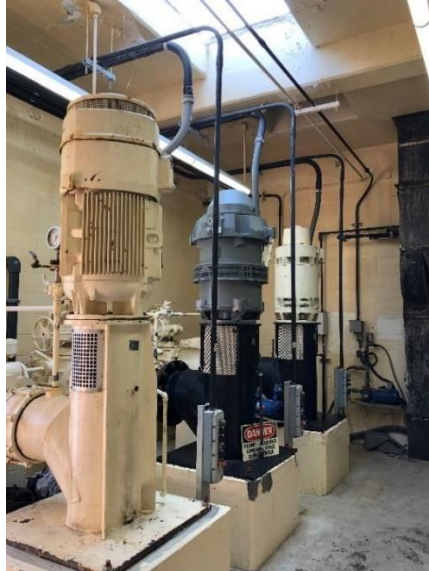
Effluent pumps 1, 2, and 3
