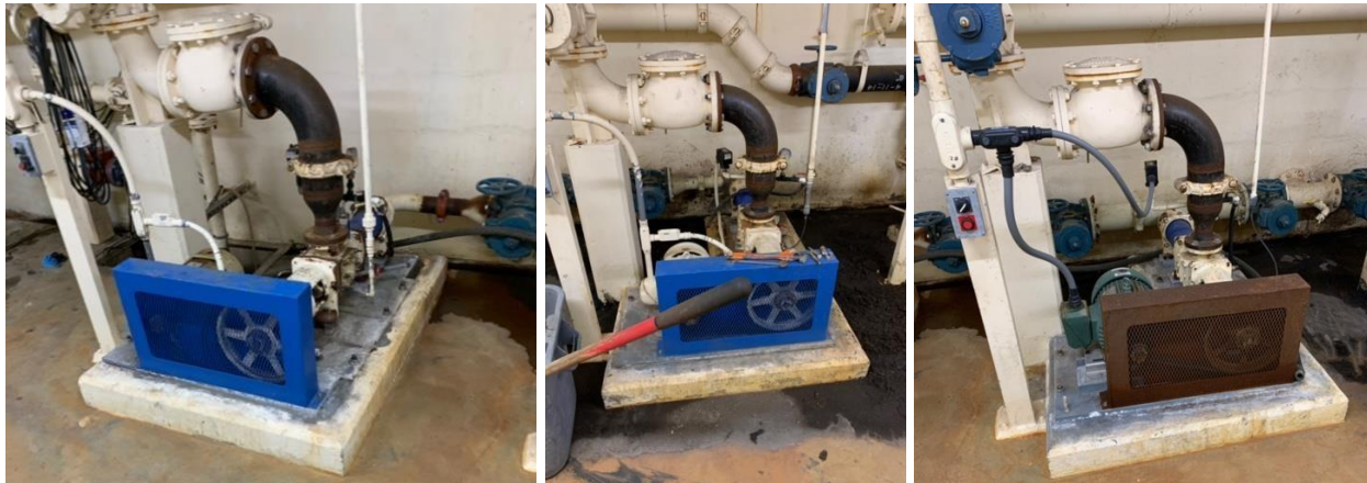
Primary Sludge Pumps 1, 2, and 3
