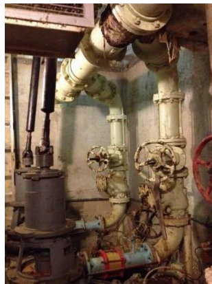
Existing Princeton Pump Station pump room
