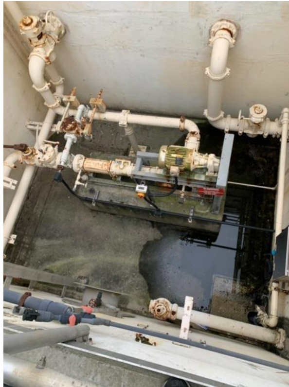
Primary scum pump and motor
