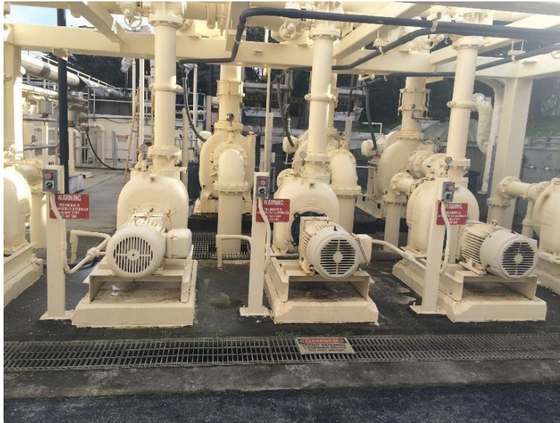
Influent pumping station
