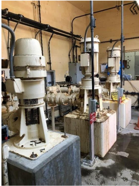
No. 3 water pumps 1, 2, and 3 (pump 4 not shown)
