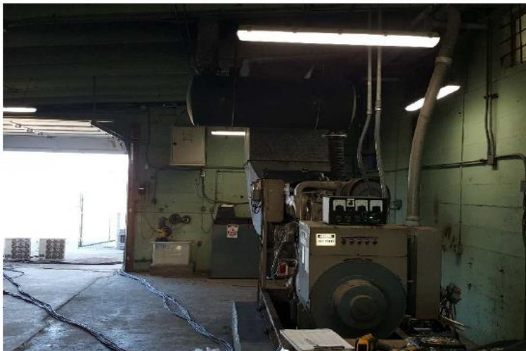
Figure B-1 Montara Pump Station Generator
