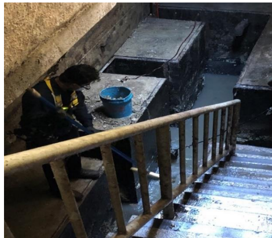
Figure B-5 Portola Pump Station Wetwell
