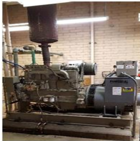
Figure B-3 Portola Pump Station-Generator
