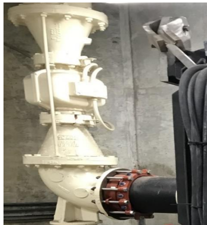
Figure B-2 Montara Pump Station Flow Meter
