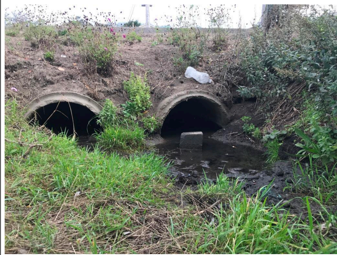
Photograph 10: Intermittent stream IS-2 and culverts running from under Obispo Road. Looking southwest from under Obispo Road. Looking north from the bank.
